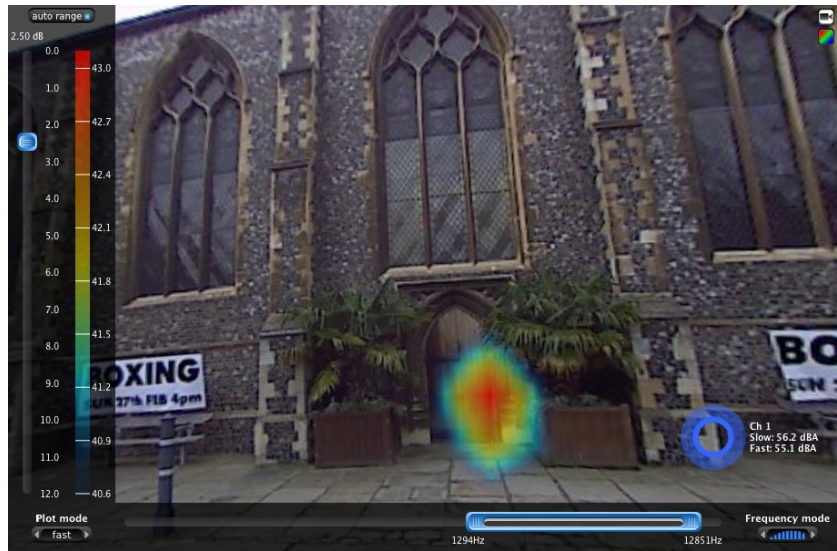
Figure 5 – Seal missing on external door
